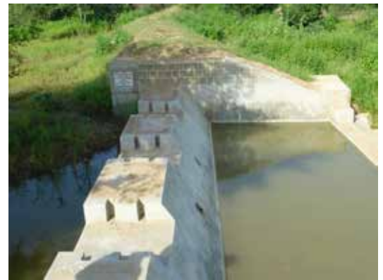
Figure 14 : Chandrapal group's check- dam ,September 2014
